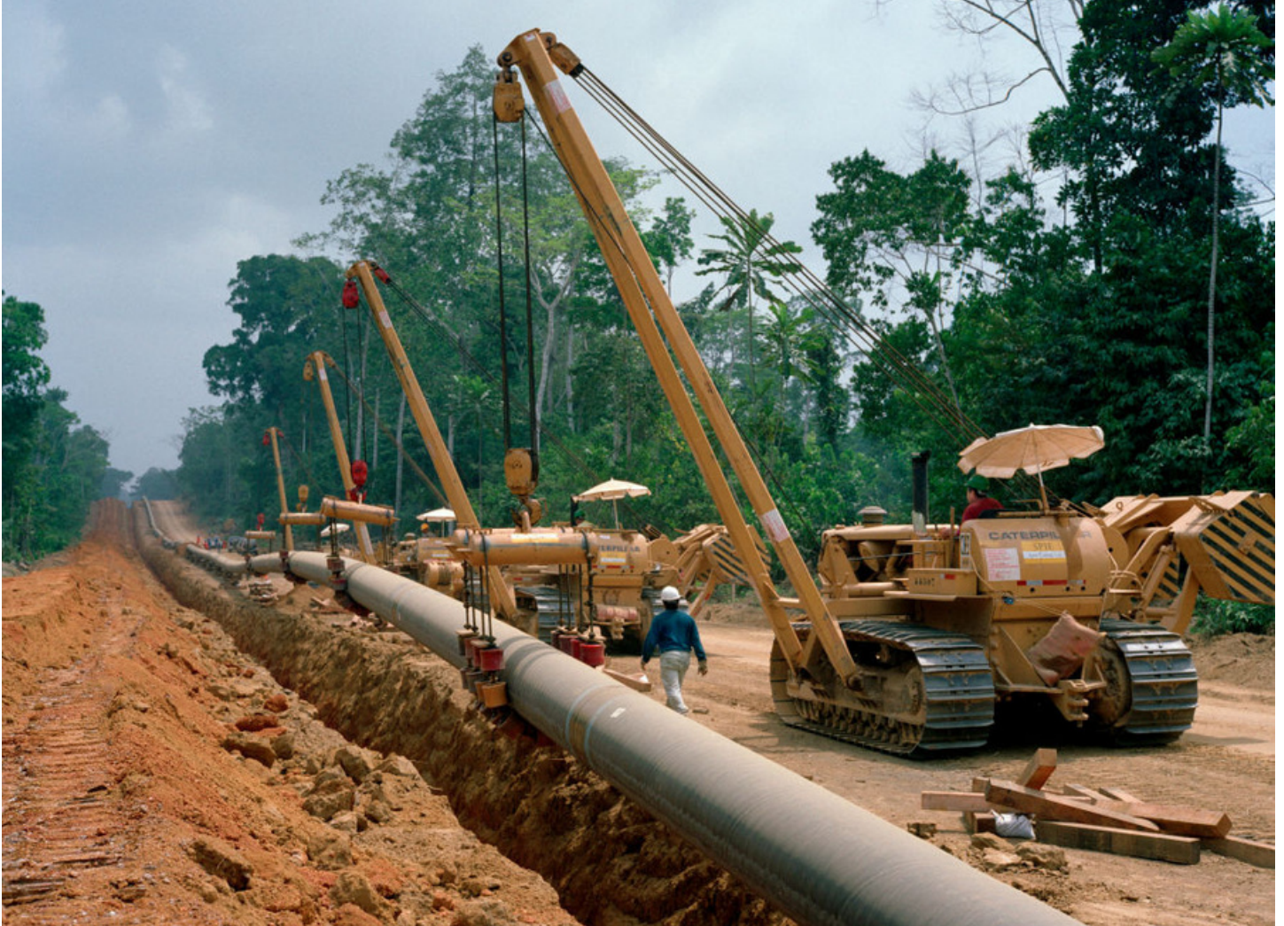
Chad-Cameroon pipeline. Source: Tom Stoddart/Getty Images
